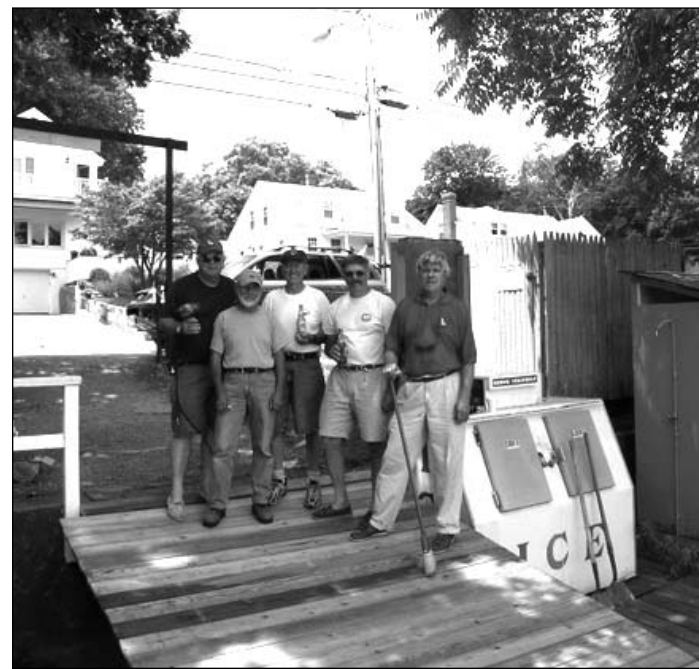
Whew!!! Having just completed the building of the new Dinghy Ramp on Saturday July 9th. Included in the picture are, left to right Eric Jones, Bevan Crighton, Jack Scaduto, Russ Carr, Bob Gibbs. Not included in the picture, but who also helped build the ramp are Guy Hannum and Chuck Wargo.
